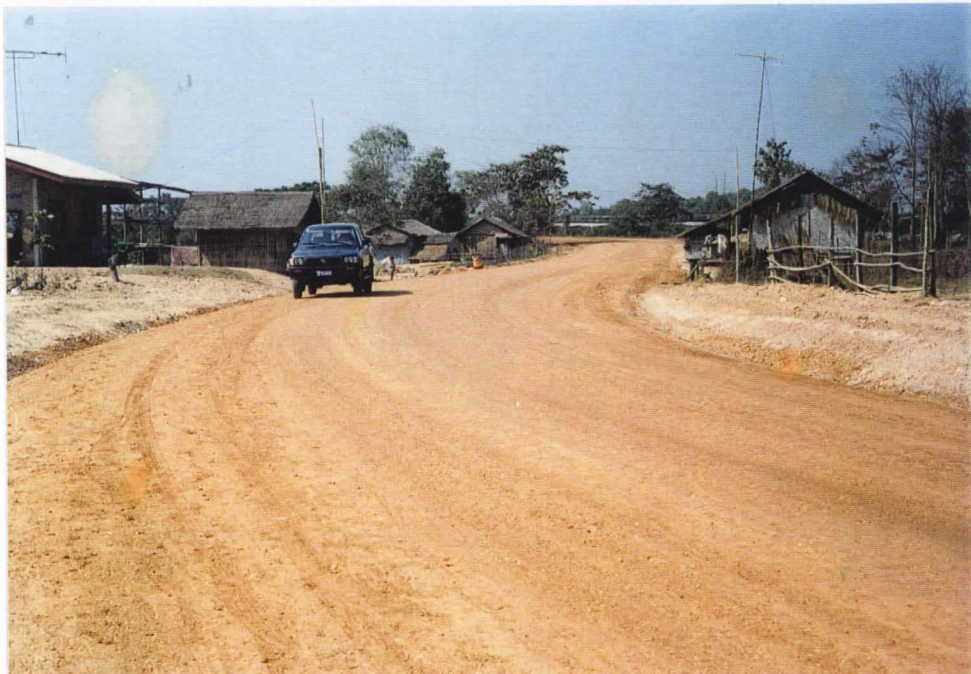
Photo 22. In this period 39 km on 5 new roads have been 60% completed for survey and design for new construction. This Photo is of the new road at Na Kha PBP.
