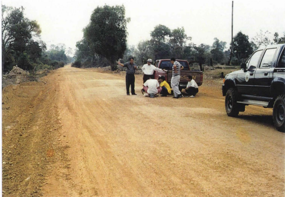
Photo 21. During this period a total of 13.7 km of roads were constructed at 3 sites. This road was at Phon Sim PBP.
