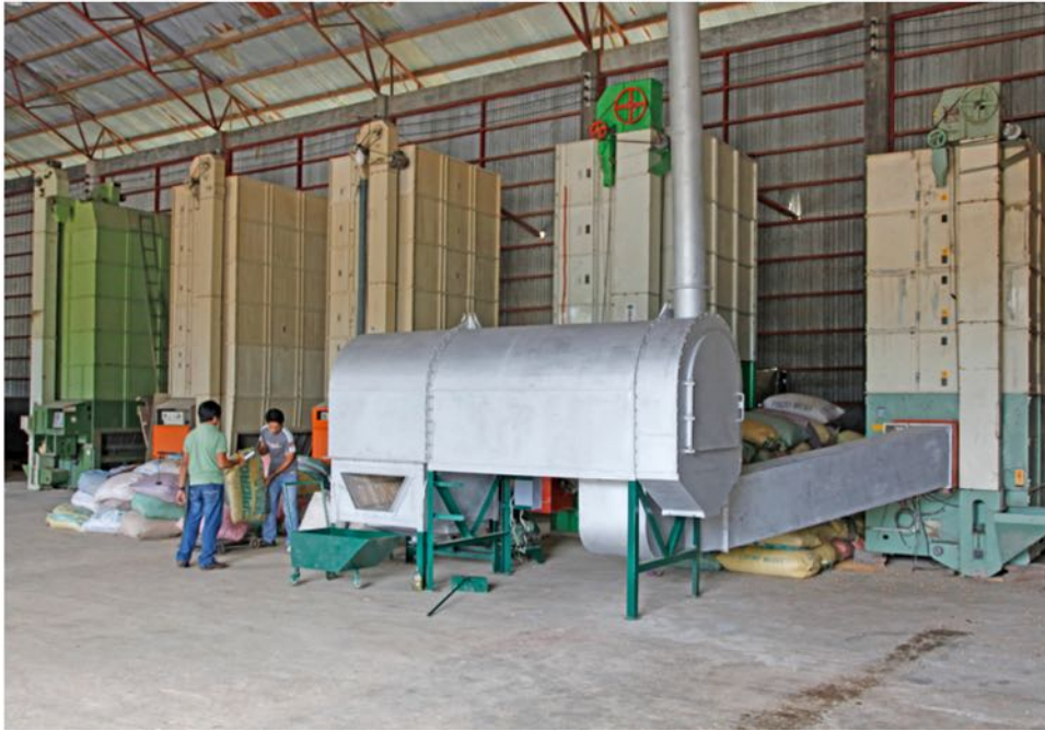
Multi-Fuel Biomass Furnace, PHilMech Design [12]
