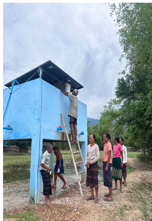
Figure 4: Solar powered pump system and water tank installed in trial village in the Attapeu ALL.
