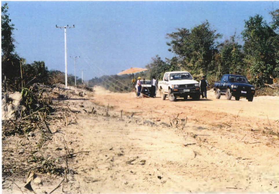
Photo 11. Three new road construction contracts were signed in this reporting period and two contractors have already mobilised and started the road works. This photo shows the start of works on the Pakngan Road in Vientiane Prefecture.
