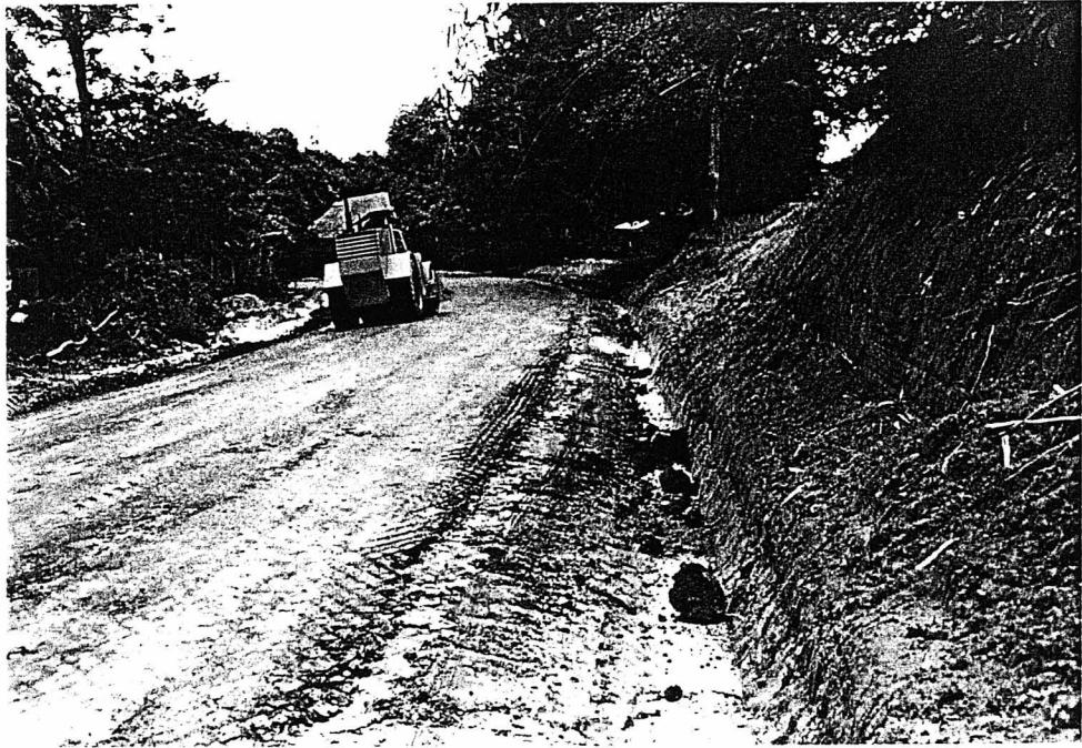
Photo 13. Road contract tender and contract documents were completed for 4 of the 5 civil works the 5th is 65% completed and will be finished in early July. Two construction contracts were started. This photo is of shows construction of the Phon Tong access road, Vientiane Province.
