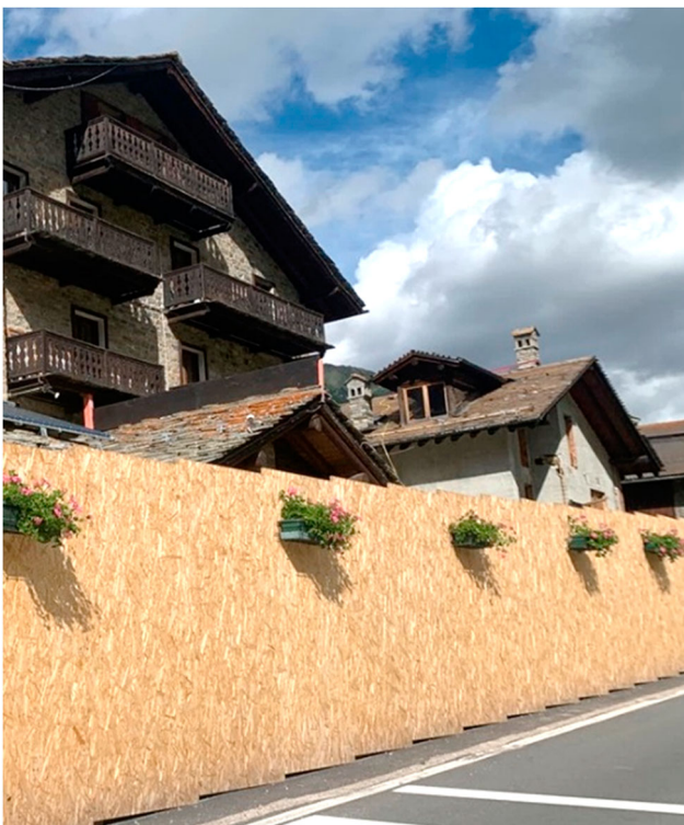
Figure 1. OSB is often used in some exterior applications such as hoarding (image Zanuttini).
