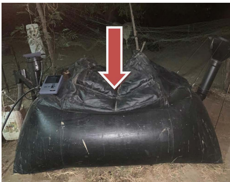
Figure 9. HBG2 tank completely emptied by uncontrolled use of biogas.
